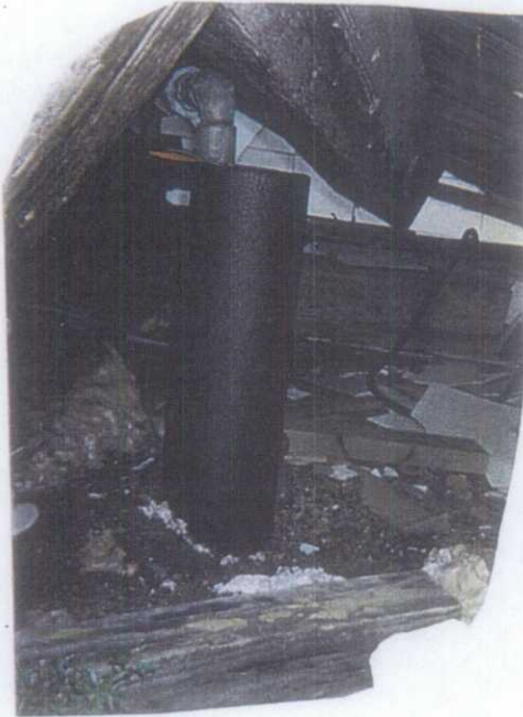
↑ WELL #1, SOUTH OF BLDG. 113
