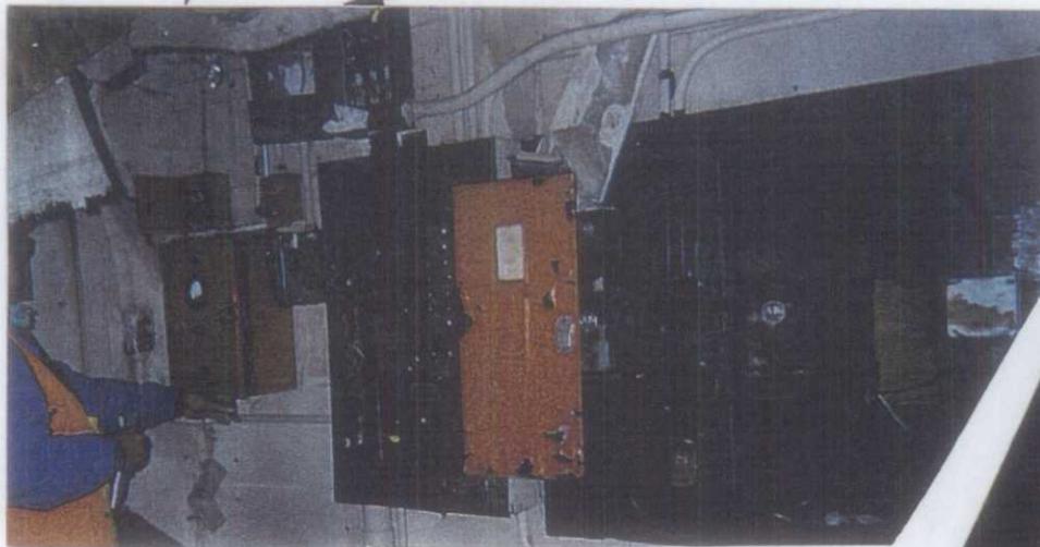
EAST WALL GROUP WASTINGHOUSE PANEL BOX- 15 BREAKERS
