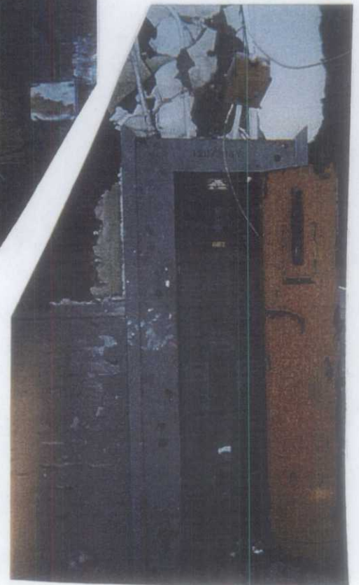
WEST WALL SWITCH BOX
