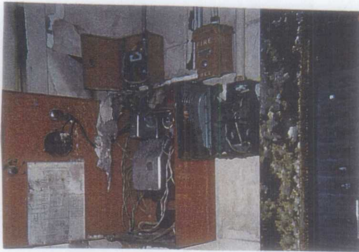
FIRE PULL, FIRE ALARM RIGHT SIDE OF MAIN GROUP
