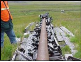
Outfall pipe and collapsed utilidor at Site 21 (2002)
