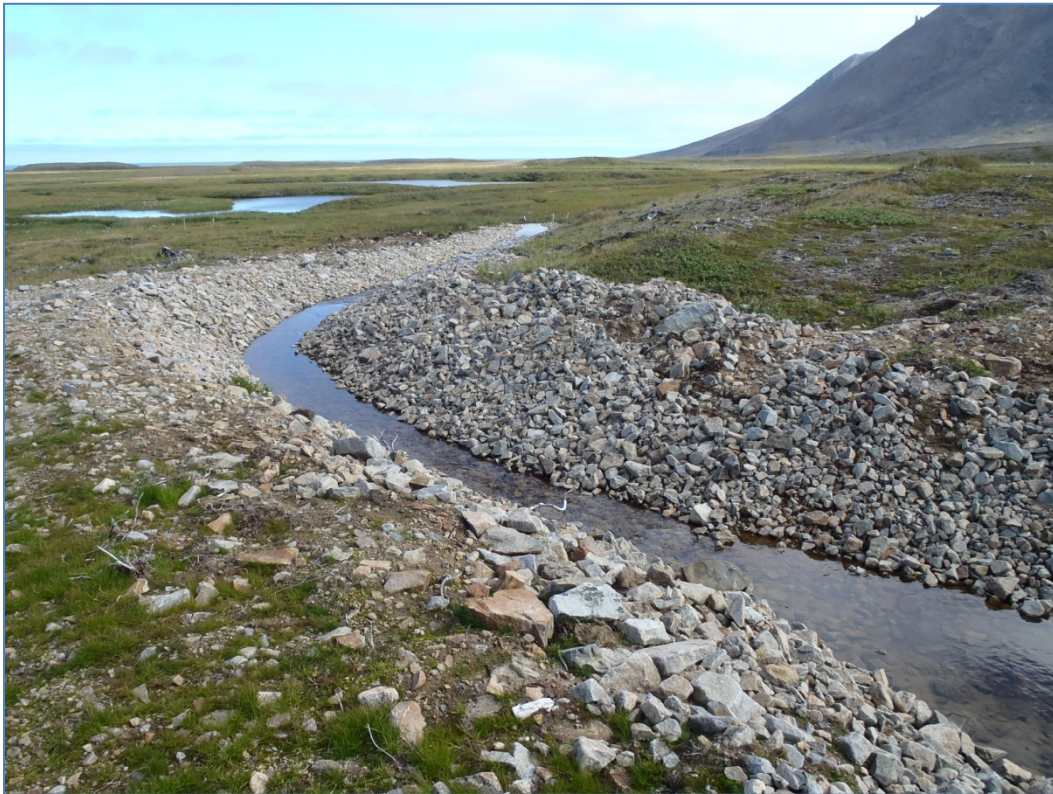
Photo 12: Site 9 Landfill – Drainage ditch operating well and in good condition, facing northeast.
