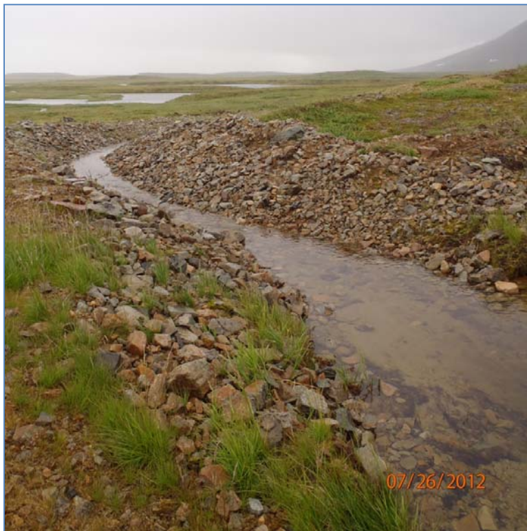
Photo 10: Site 9 Landfill – Pond outlet ditch in good condition and operating efficiently, facing northeast.
