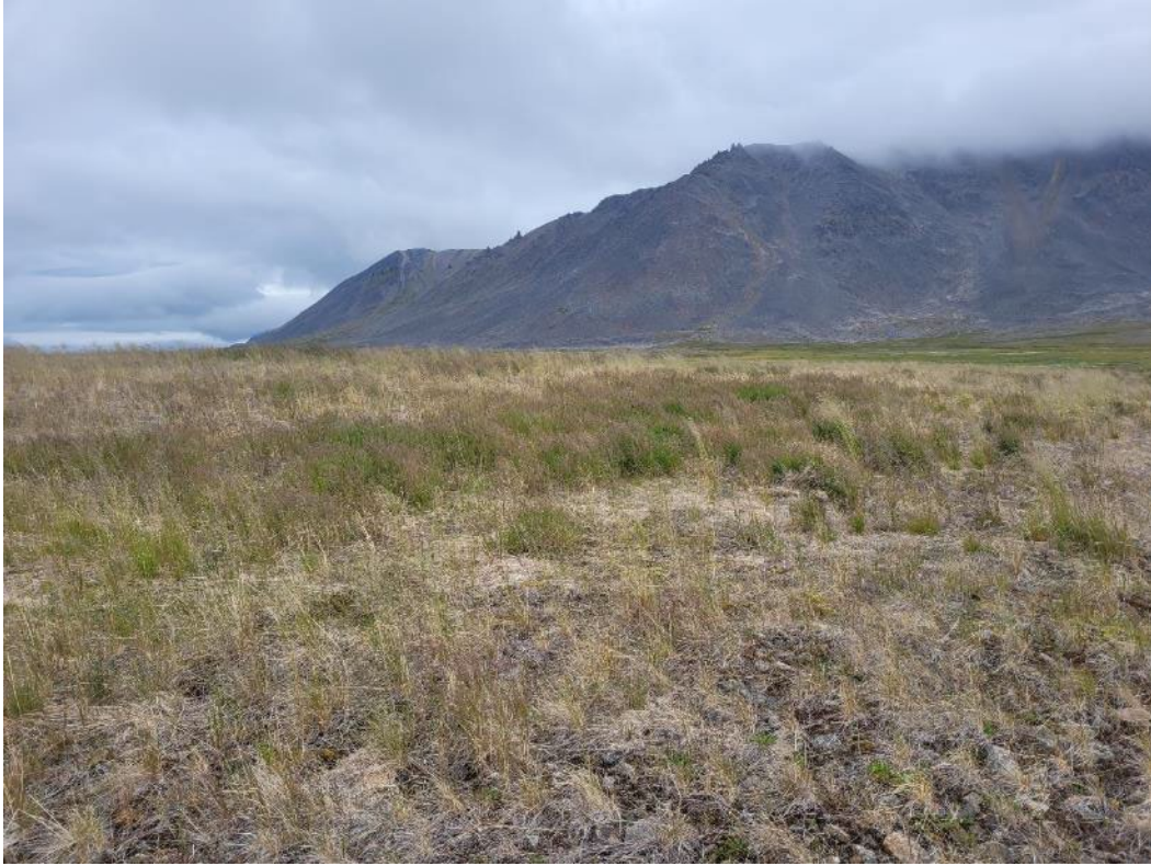
Photo 10: Vegetation growing on slope of landfill cap looking SE
