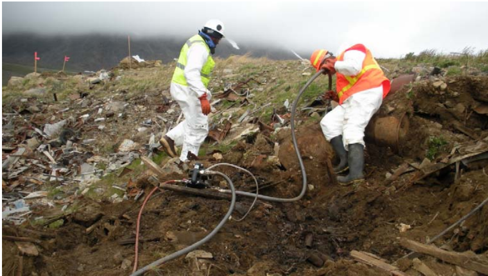
Photograph 3. Field crew pumping liquid out of a corroded drum in the landfill.
