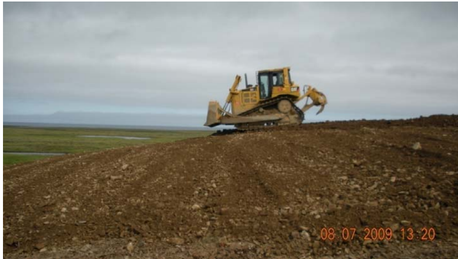
Photograph 5. Laying down and track-walking 6-inch lifts for a minimum of a 24-inch landfill cap.
