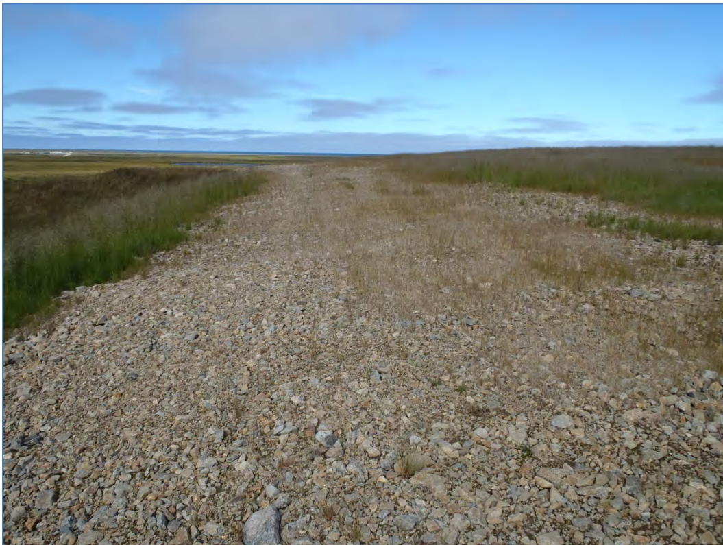
Photo 10: Site 7 Landfill – South slope of landfill, facing northwest with camp in background.
