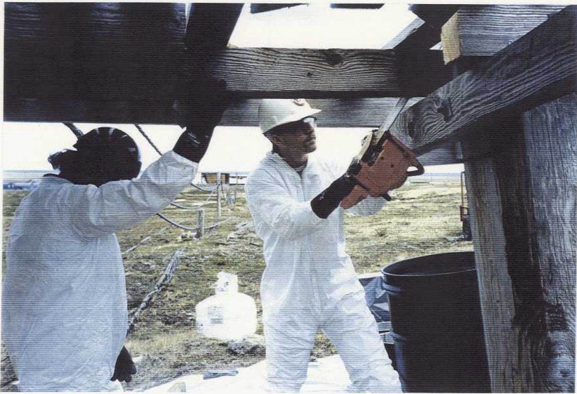
Fig. 3.31 Removal of oil-stained timbers on transformer platform viewed northwesterly along Power and Communications Line Corridor on 7/11/94 at Northeast Cape, St. Lawrence Island, Alaska. Photographed by Chuck Heath, Northwest EnviroService, Inc. on Contract DACA85-93-C-0048.
