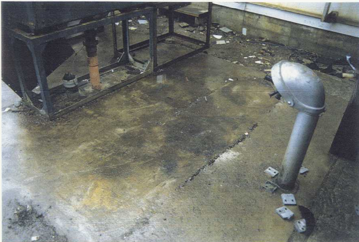
Fig. 3.4 Stained floor in Building 110 which previously housed transformers and switches. Viewed in easterly direction. Photo taken at Northeast Cape, St. Lawrence Island, Alaska on 7/20/94 by Chuck Heath, Northwest EnviroService, Inc. on Contract DACA85-93-C-0048.
