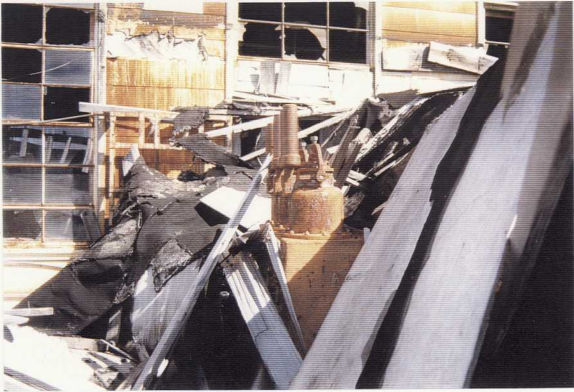
Fig. 3.1 Collapsed roof on transformer room of Bldg. 110 viewed easterly on 9/4/93 at Northeast Cape, St. Lawrence Island, Alaska. Photographed by Larry Wilkinson, Northwest EnviroService, Inc. on contract DACA85-93-C-0048.
