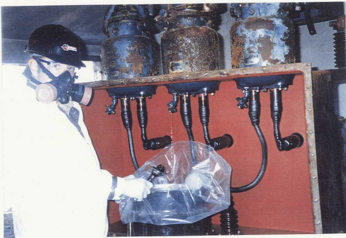
Fig. 3.8 Switch being drained inside Building 110 viewed northeasterly at Northeast Cape, St. Lawrence Island, Alaska on 7/18/94 by Michael Naquin, Northwest EnviroService, Inc. on Contract DACA85-93-C-0048.
