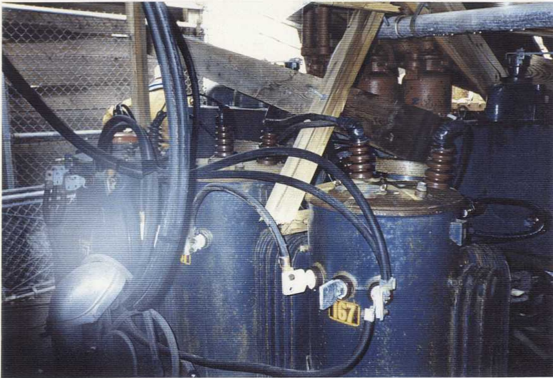
Fig. 3.3 Western set of switches with first set of transformers under collapsed roof at Building 110 viewed northeasterly and photographed by Larry Wilkinson, Northwest EnviroService, Inc. on 9/4/94 at Northeast Cape, St. Lawrence Island, Alaska on Contract DACA85-93-C-0048.
