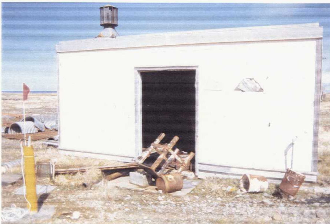
Fig. 3.22 Western entrance to Paint and Dope Storage Building with new sampling well marked with red flag, viewed easterly on 7/6/94. Photographed at Northeast Cape, St. Lawrence Island, Alaska by Larry Wilkinson, Northwest EnviroService, Inc. on Contract DACA85-93-C-0048.
