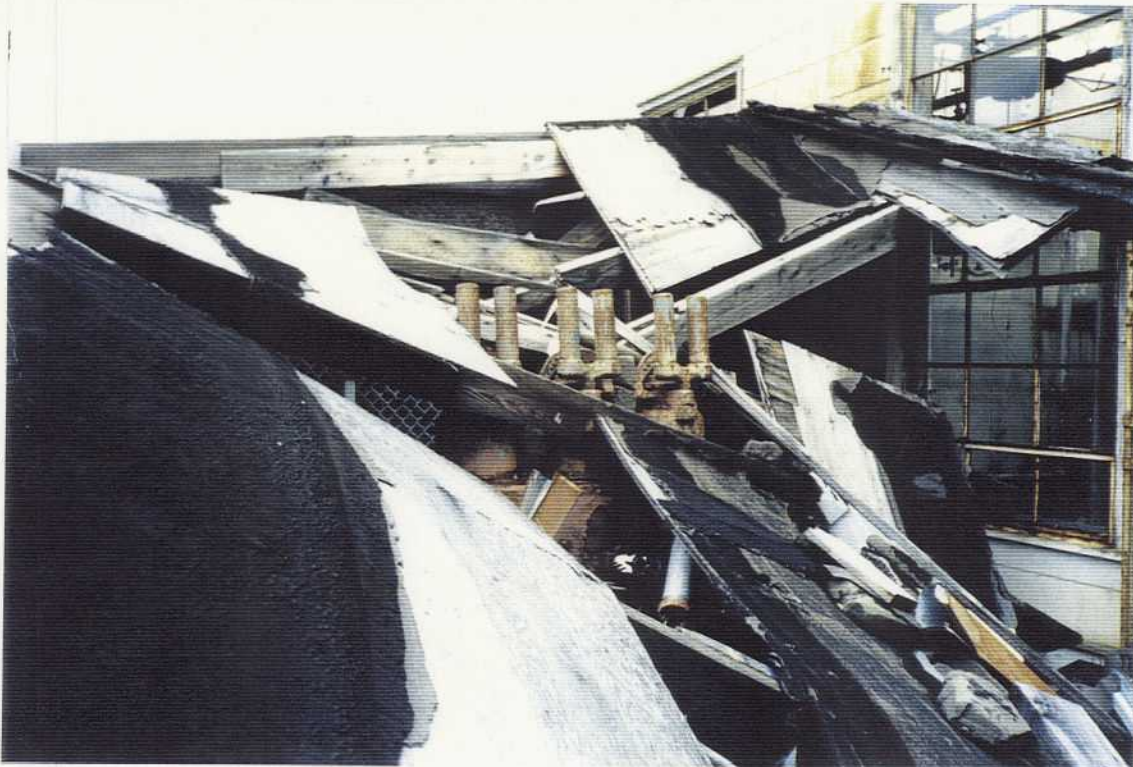
Fig. 3.9 Western set of switches under collapsed roof at Building 110 viewed westerly at Northeast Cape, St. Lawrence Island, Alaska on 9/4/93 by Larry Wilkinson, Northwest EnviroService, Inc. on Contract DACA85-93-C-0048.
