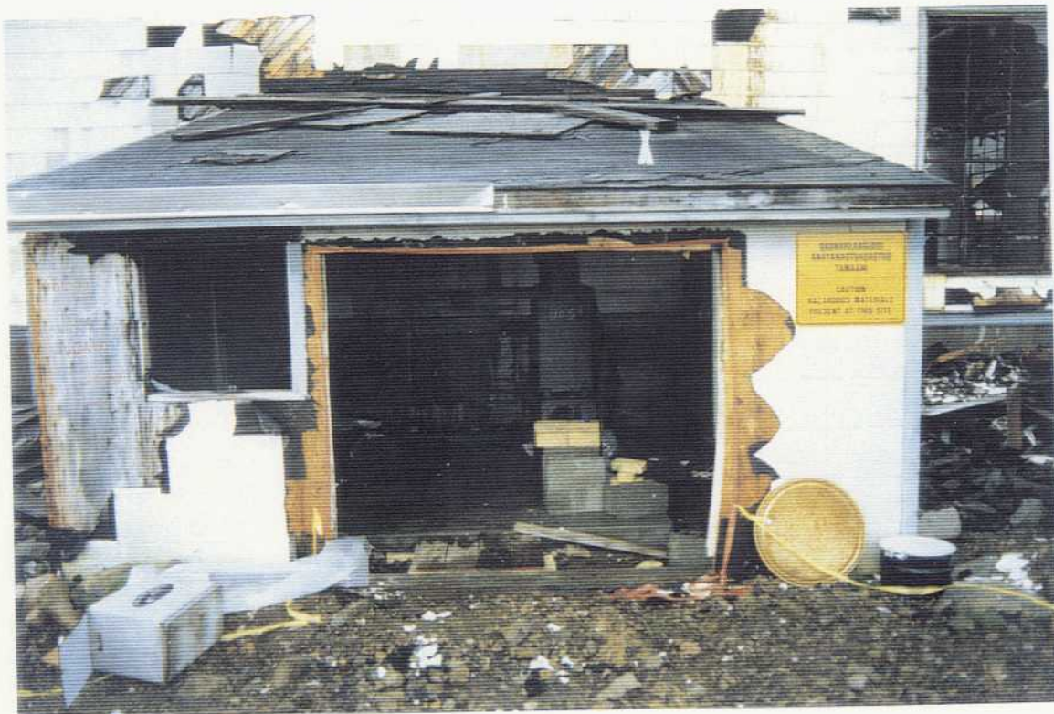
Fig. 3.12 New doorway on transformer room; viewed southeasterly on 7/16/94 at Northeast Cape, St. Lawrence Island, Alaska. Photographed by Chuck Heath, Northwest EnviroService, Inc. on Contract DACA85-93-C-0048.
