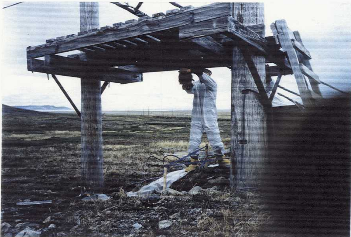
Fig. 3.32 Removal of oil-stained timbers over oil-stained pit from which soil was excavated. Viewed westerly along Power Corridor on 7/11/94 at Northeast Cape, St. Lawrence Island, Alaska. Photographed by Chuck Heath, Northwest EnviroService, Inc. on Contract DACA85-93-C-0048.
