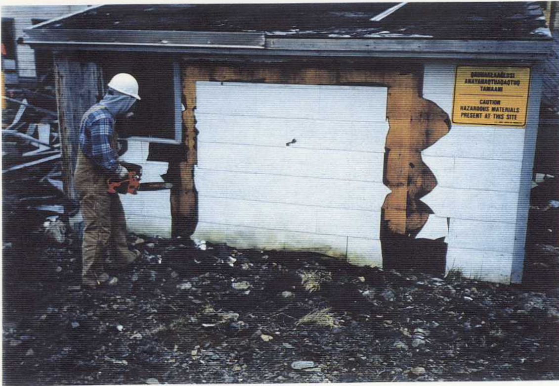
Fig. 3.11 Transformer room redesign in progress following asbestos shingle relocation; viewed northeasterly on 7/16/94 at Northeast Cape, St. Lawrence Island, Alaska. Photographed by Chuck Heath, Northwest EnviroService, Inc. on Contract DACA85-93-C-0048.
