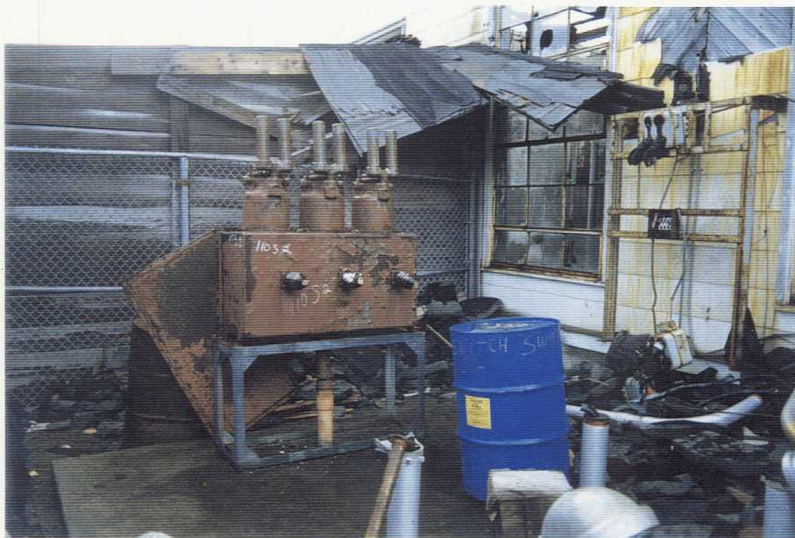
Fig. 3.10 Western set of switches with roof removed at Heat and Electric Power Building at Northeast Cape on St. Lawrence Island, Alaska viewed northerly and photographed on 7/20/94 by Chuck Heath, Northwest EnviroService, Inc. on Contract DACA85-93-C-0048.
