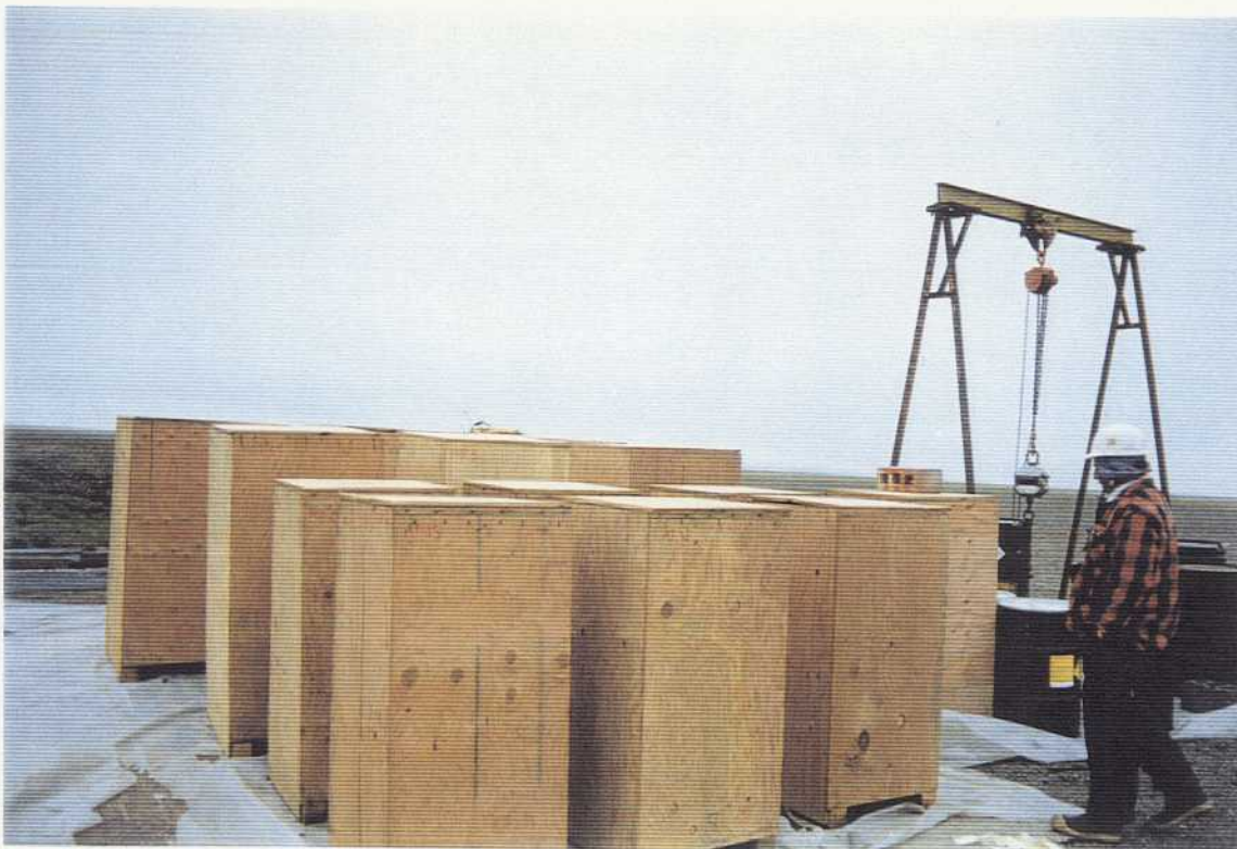
Fig. 3.37 Drained and Crated PCB transformers awaiting labels and markers at Northeast Cape on St. Lawrence Island, Alaska. Viewed southerly on 7/30/94. Photographed by Larry Wilkinson, Northwest EnviroService, Inc. on Contract DACA85-93-C-0048.
