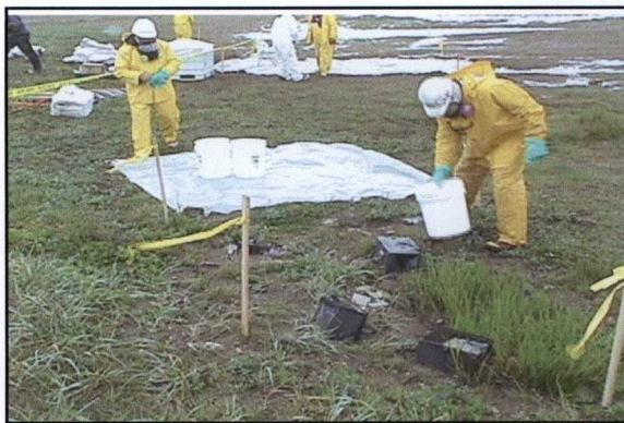
Photo 47: Workers in Level "C" PPE remove batteries and dried paint at Site 12.
