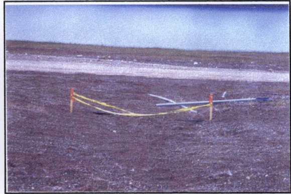
Photo 32: Energized power cable for runway lights exposed at Site 8. (Metal debris suspended near power cable.)
