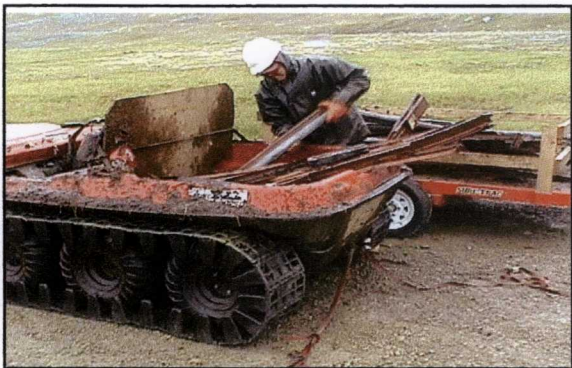
Photo 17: Worker transferring metal debris from Argo to wagon for transportation to weighing station at Site 8.
