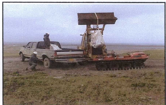
Photo 18: Backhoe removing supersack containing Site 4/Area 4A debris from Argo to pickup truck.
