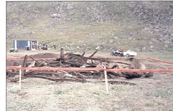
5. SAFETY FLAGGING AROUND EXCAVATED DEBRIS
